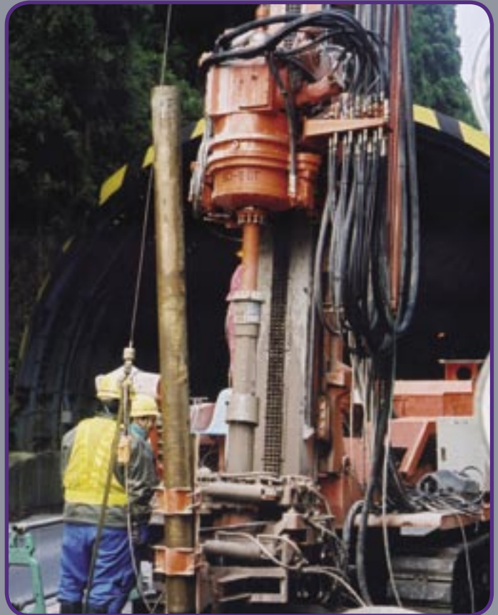
■ Drilling for the installation of geo-exchange tubing at a highway tunnel entrance.
