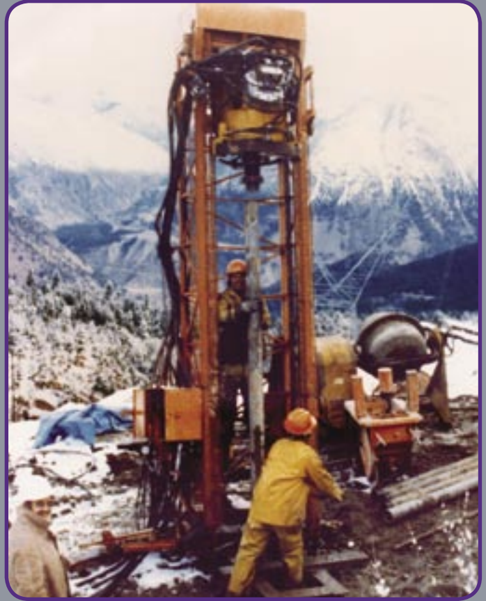
■ Installing combination micro pile and tension anchors for hydro-electric transmission towers in unstable ground conditions.
